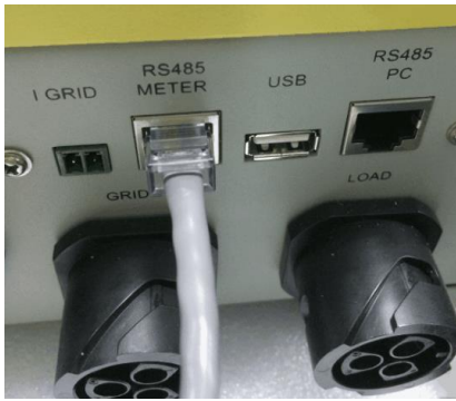
Figure3-19 Wire connection of smart meter
